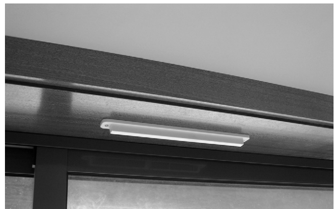
Fig. 3. Self-regulated inlets fitted above the windows.
