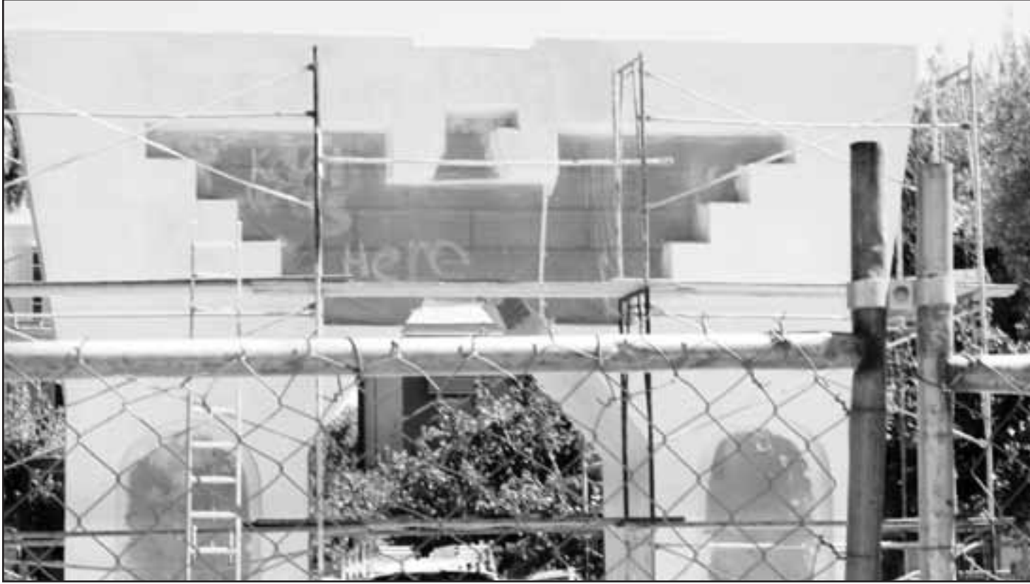
The site of the Cesar E. Chavez Monument remains surrounded by chain-link fences.
