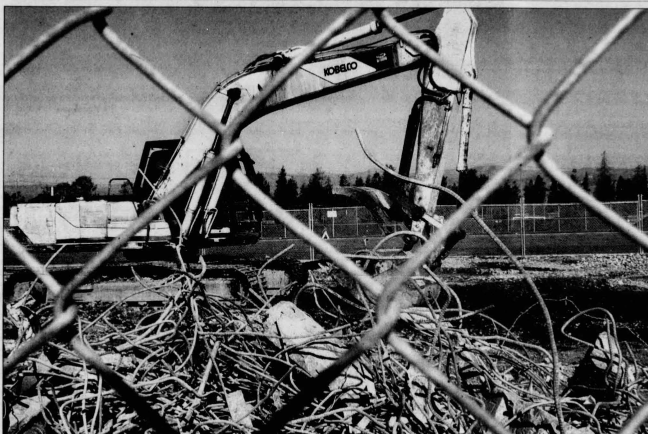
ABOVE: Workers sift through the huge pile of debris at Bud Winter Field on the corner of Seventh and Alma streets. The debris came from the demolition of Moulder, Markham and Allen halls. RIGHT: Ricky McCoy, a sophomore sociology major, ran beside the huge pile of debris on Bud Winter Field at Seventh and Alma streets Thursday. McCoy said the strong smell coming from the refuse keeps his visits short.
