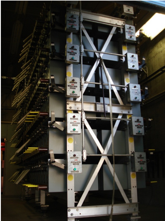
Figure 2.2. The 6-tier capacitor capacitance bank.
