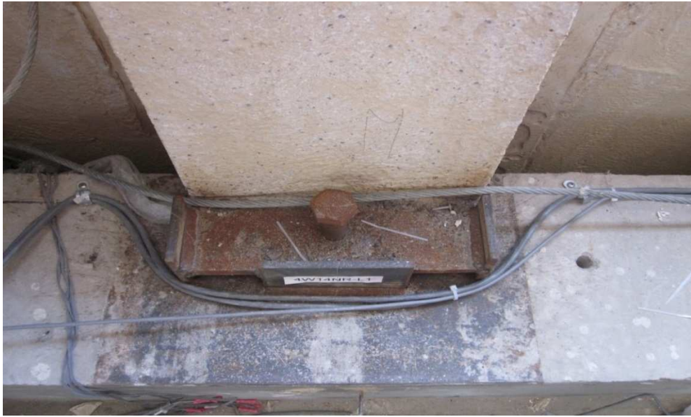
Figure 2. Photograph of the bearing connection at UCSD (personal communication, June 2013) (reprinted with permission from Kurt McMullin).
