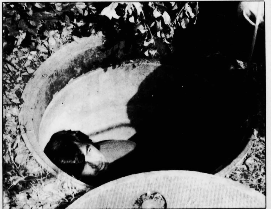
John Johnson, who works for Telephone Plant near Clark Library. He is installing a new fiber Construction Corp., looks up from a manhole optics backbone.
