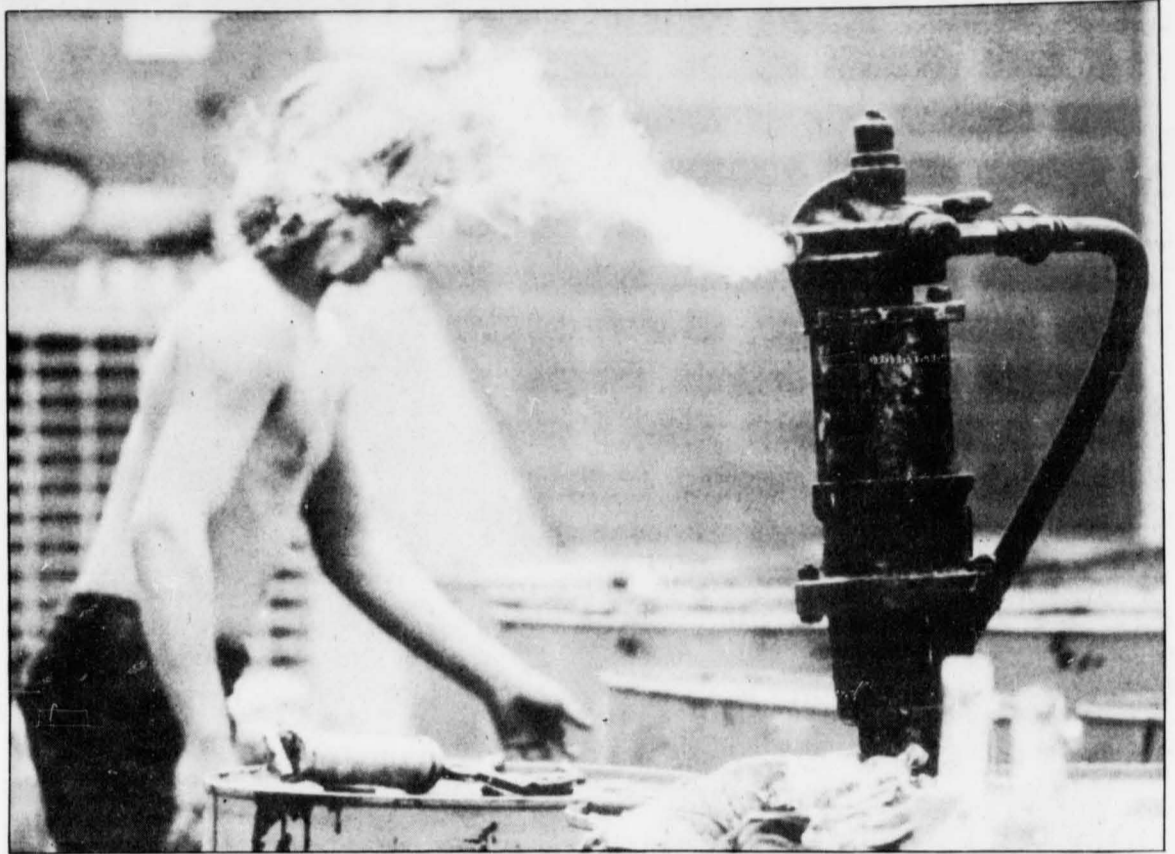
Students living in the Hoover, Royce and Washburn resident dorms have been waking up every morning to the loud banging noise of this air pump. The pump is used to load tar on the rooves of the dorms, which are being resurfaced. The roof repair project, which costs approximately $170,000, is being funded by the public works portion of the CSU budget. Brigham Taylor Construction Company was awarded the contract.
