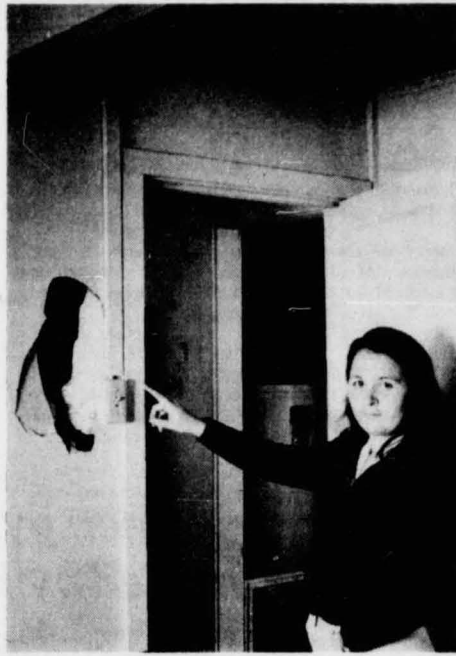
photo by Linda Colburn Bernice Mestaz, also a Spartan City resident, points out a large hole in the wall that was there when she moved into her apartment. Residents say most repairs are made promptly by Auxiliary Enterprises maintenance crews.
