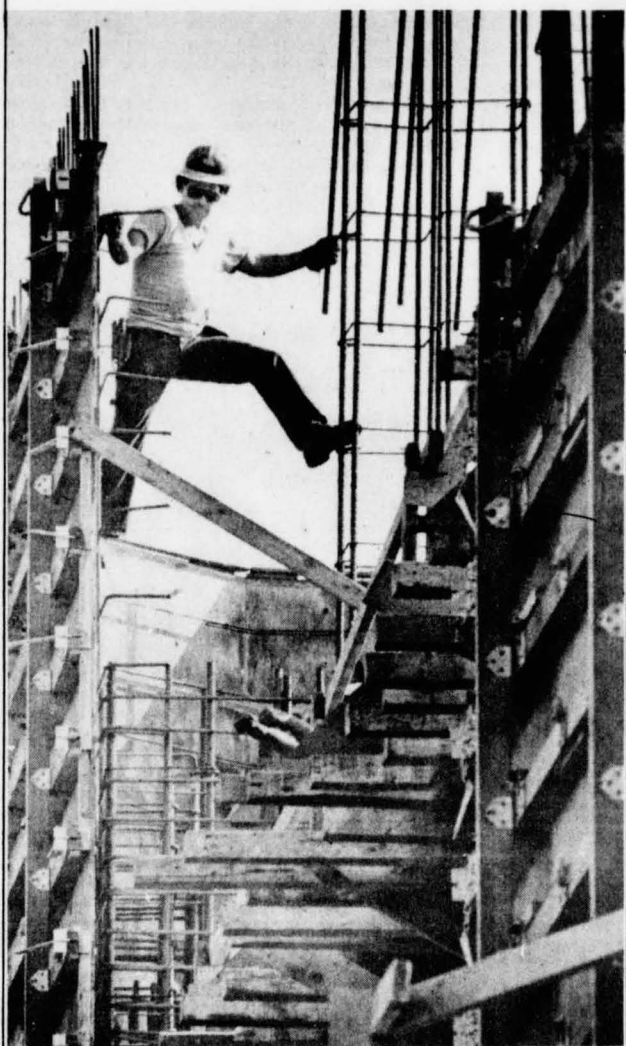
Ironworker Manuel Carrillo waits for some iron to add to the side of the new library.
