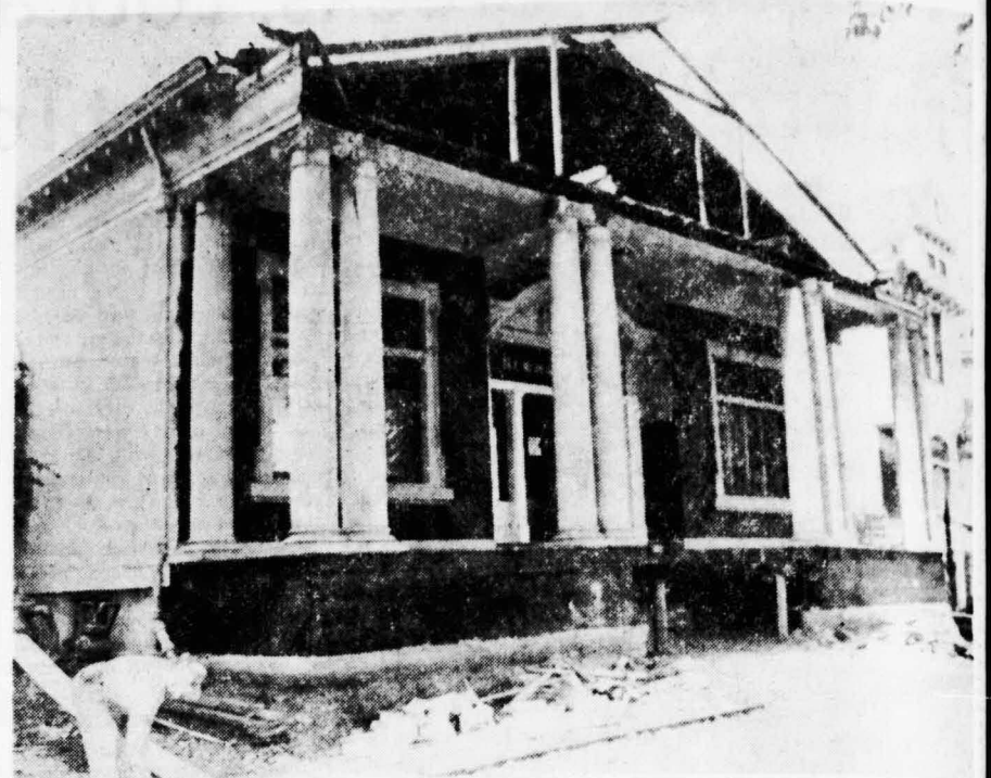
FACE LIFTING—The Newman Club Building, located at 79 S. Fifth St. and meeting place for Catholic students at SJS, is being repaired for the first time since its construction in 1913. The total cost of the repair job is expected to be $40,000. The new repairs call for a modernized front, several classrooms, a new kitchen, im-
