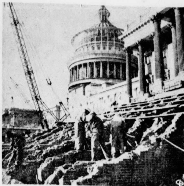
MAKING WAY for construction on subway terminal underneath, workmen tear down steps of Senate wing of Capitol in Washington. Steps will be rebuilt of granite.
