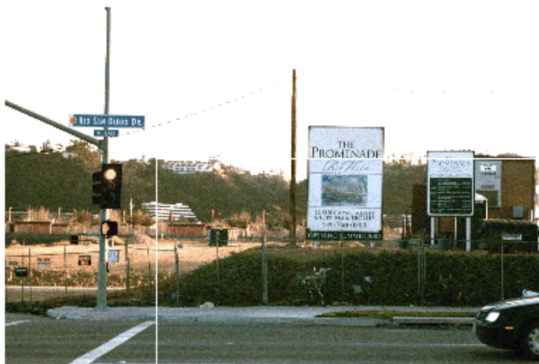
Figure 4-5: Mixed-Use and Transit-Oriented Development combined-- a view of the Promenade, a complex with retail below and apartments above, under construction in December 2000.
