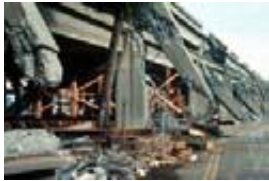
Loma Prieta damage to Cypress Structure, Oakland, CA
