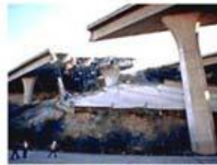
Highway vulnerability to Northridge Earthquake
