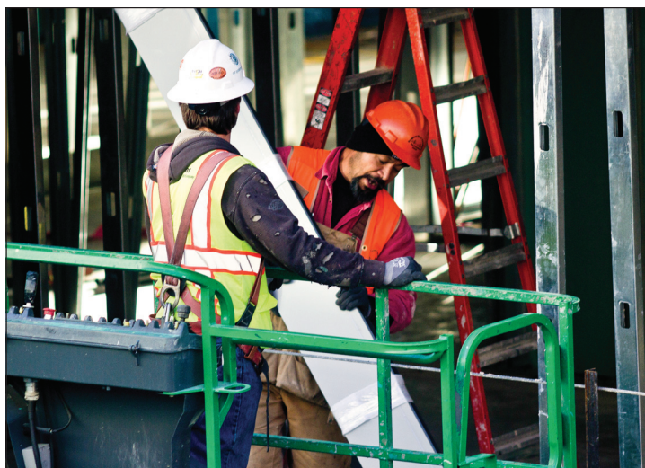
Two construction workers work together to position a piece of sheet metal while working on the Student Union Thursday Jan. 31, 2012. The Student Union construction is scheduled to be completed January 2014. Photo by Codi Mills / Spartan Daily
