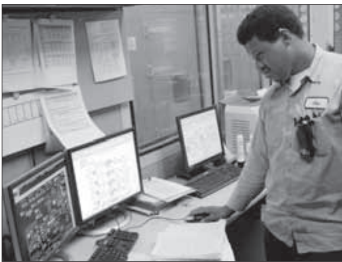
Otis Mcinnis, power plant operator for Facilities Development and Operations, demonstrates the computer system used to control and monitor the heating and cooling system that serves the entire campus on Monday. KEVIN HUME / SPARTAN DAILY
