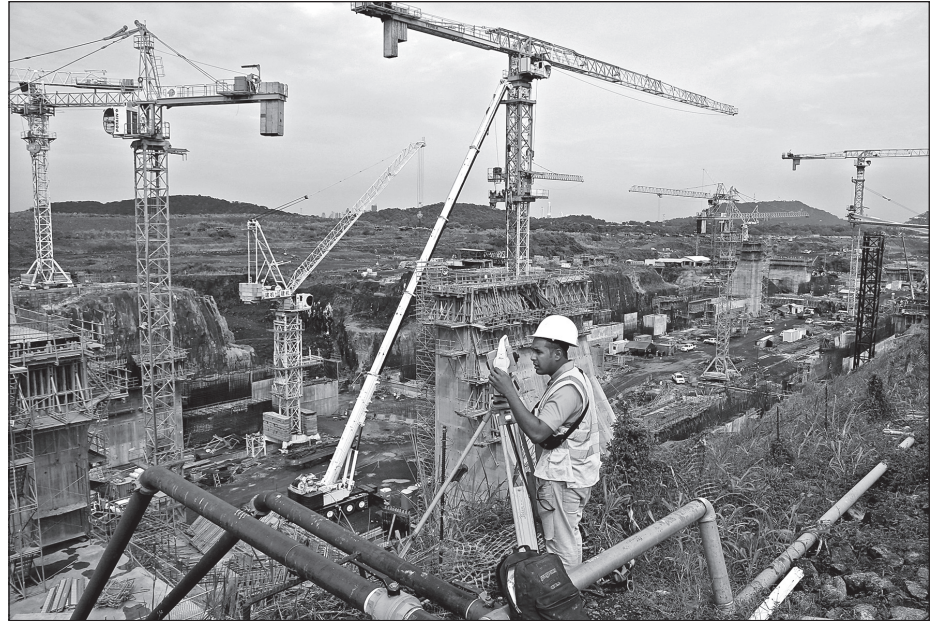
Construction of the new set of locks is 24-hour operation as Panama works towards 2015 completion date. The original Panama Canal was considered the "moon shot" of its time. The Panama Canal expansion may be the Mars trip of today. Photo by Carl Juste / MCT.
