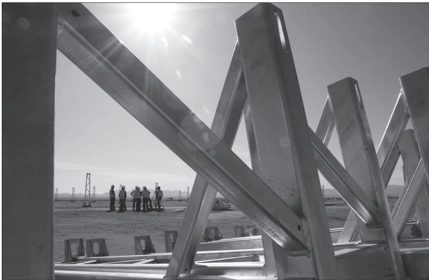
Workers are seen through the parts of pylon that are being installed to hold huge mirrors at Genesis Solar Energy Project located approximately 25 miles west of the city of Blythe, Calif., Jan. 31. The project is an undeveloped area of the Sonoran Desert on lands managed by the Bureau of Land Management. Photo courtesy of Irfan Khan / MCT
