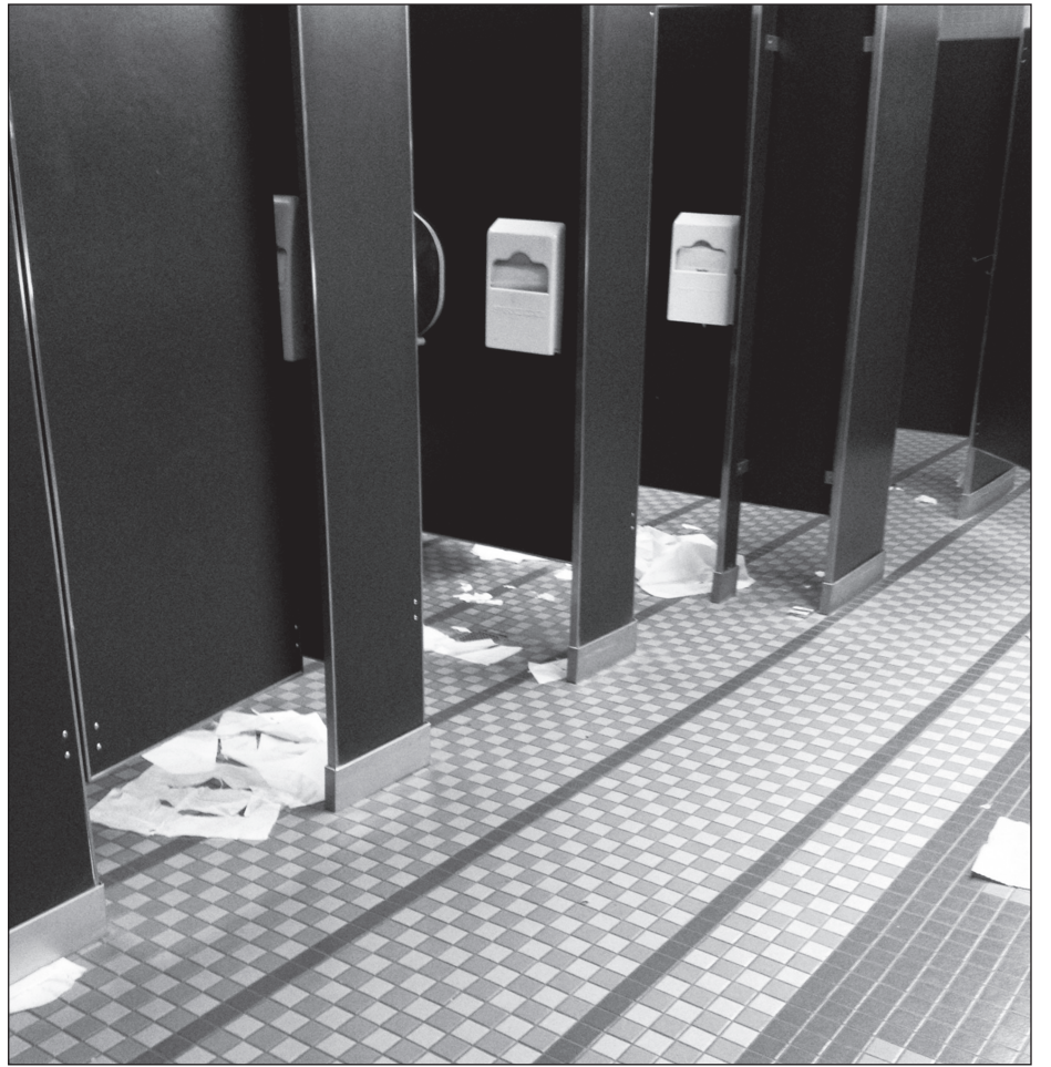
The women's bathroom on the first floor of Boccardo Business Complex. Photo by Melanie Martinez / Spartan Daily
