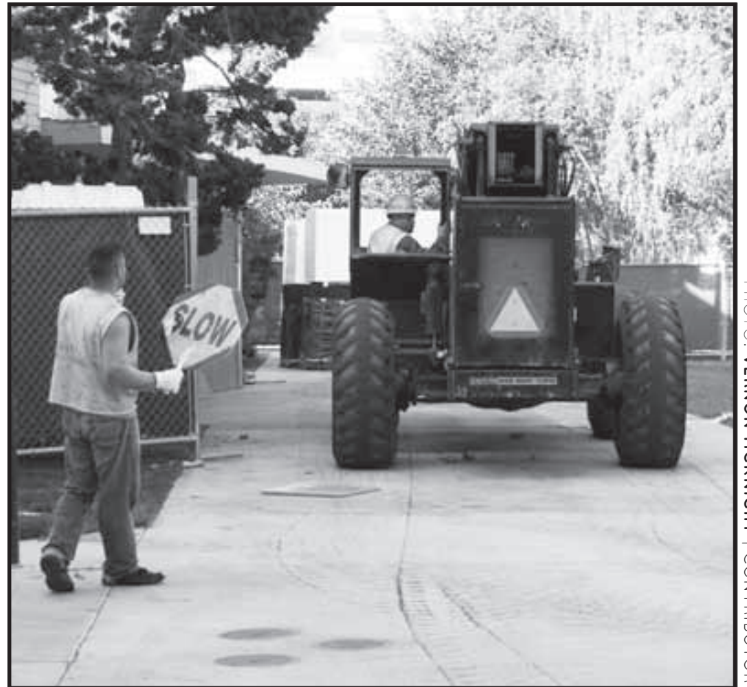
The walkway between the University Technology Services building and Dudley Moorhead Hall has been closed since last week for construction.
