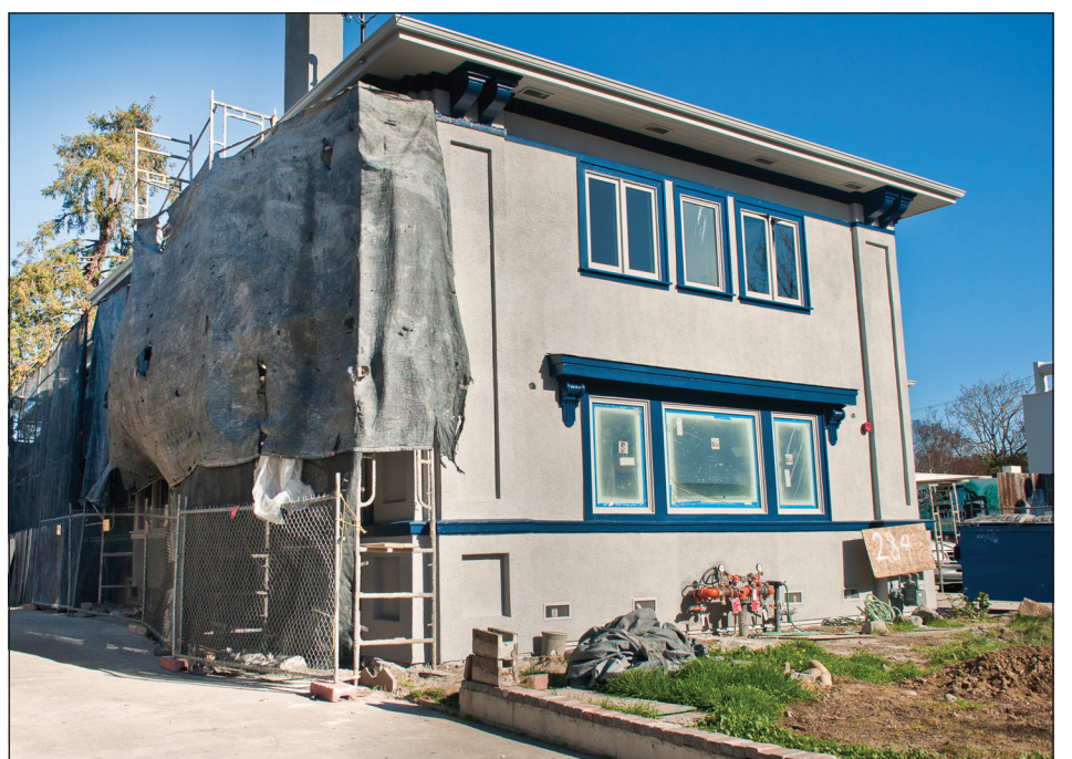
Construction on the Kappa Sigma house is set to be complete tomorrow. Basil Sar / Spartan Daily
