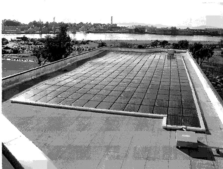
Closeup of the PV System on the City Hall in Vallejo, Californi
