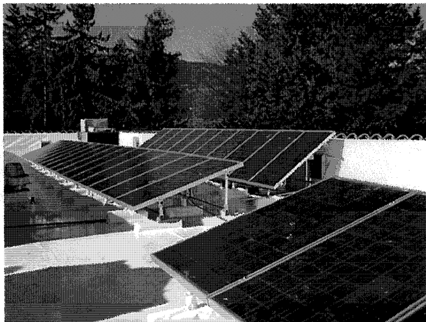
5.5 kW PV System on Civic Center in Ukiah
