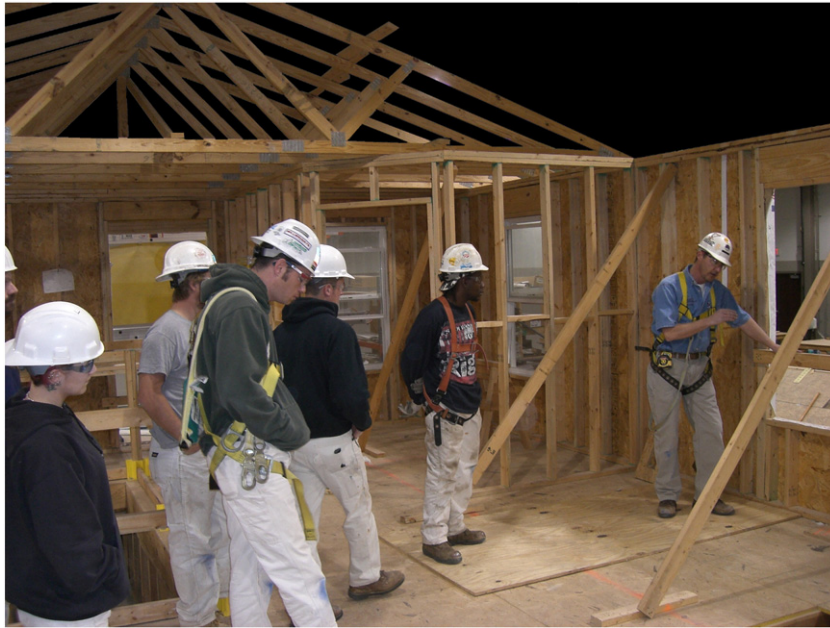
Fig. 2. Mock home demonstrates fall safety hazards and fall protection methods.
