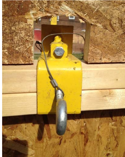
Figure 6 – Notching of wall scaffold bracket.
