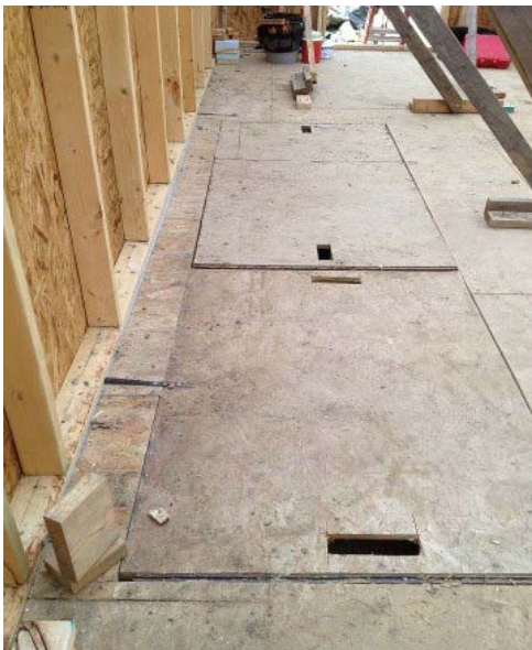
Figure 9 – Reusable sections of stair opening covers. Note: handle holes should be covered.
