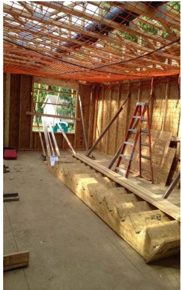
Figure 2 – Safety net spans the width of the home.
