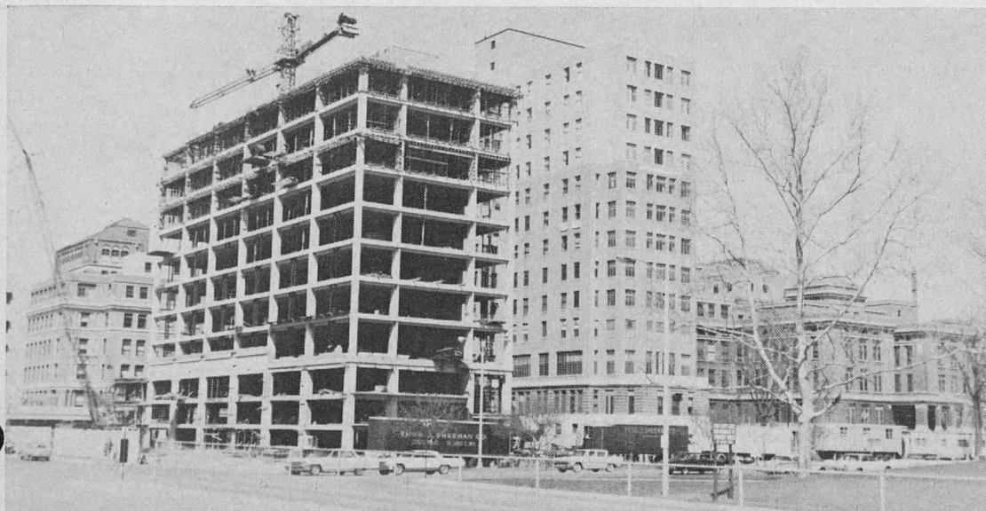
Construction work continues on the Queeny Tower building which will dominate the Medical Center upon completion. Concrete work will be finished in July. Brick work has been started and has reached the sixth floor of the structure, which will tower 18 stories when completed in August of next year.
