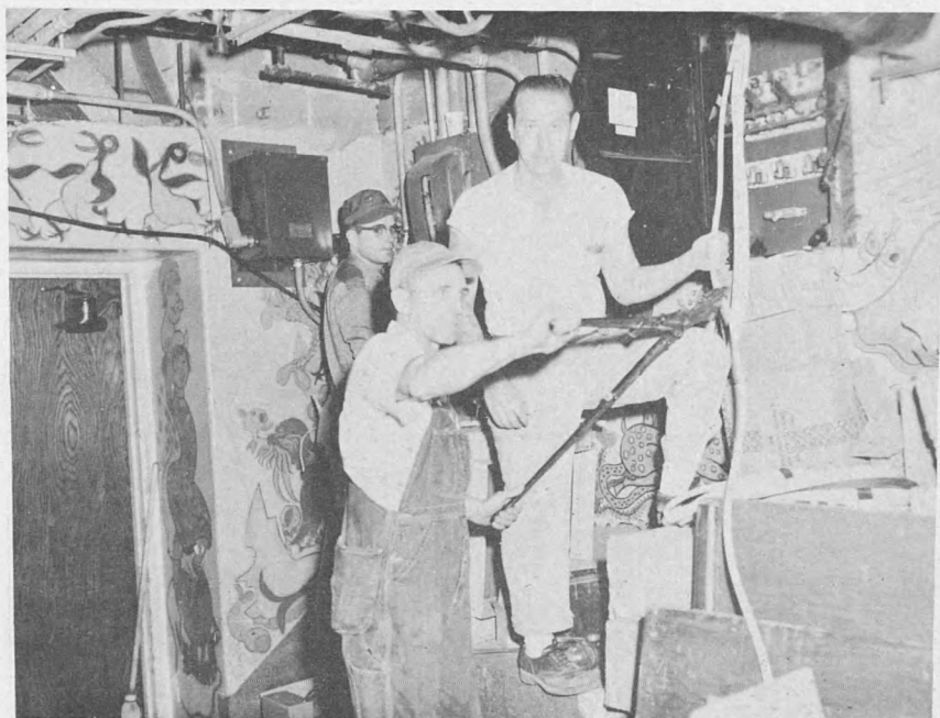
Shown above are electricians rewiring fourth floor Operating Room Switch Panels: Left rear is Charles Longo, center front is Leylan Creed, and at right is Robert Spradlin.
