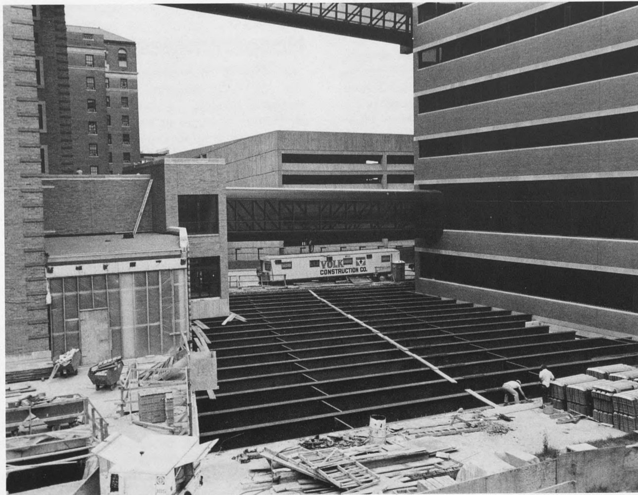
Construction on the new emergency facilities has included the unusual task of expanding Renard bridge. The project will be completed in about one year.
