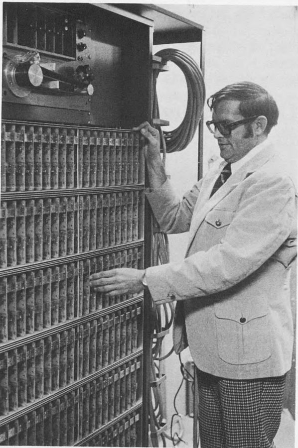
George Voyles, director of telecommunications, inspects installation of new Centrex telephone system for patient rooms. The unit shown is the Hospax addition to the system.
