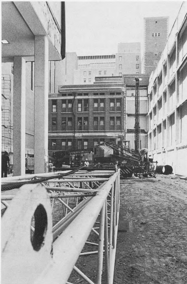
An empty space remains where the number four building in the hospital was previously located. A new service building will be built on the site.
