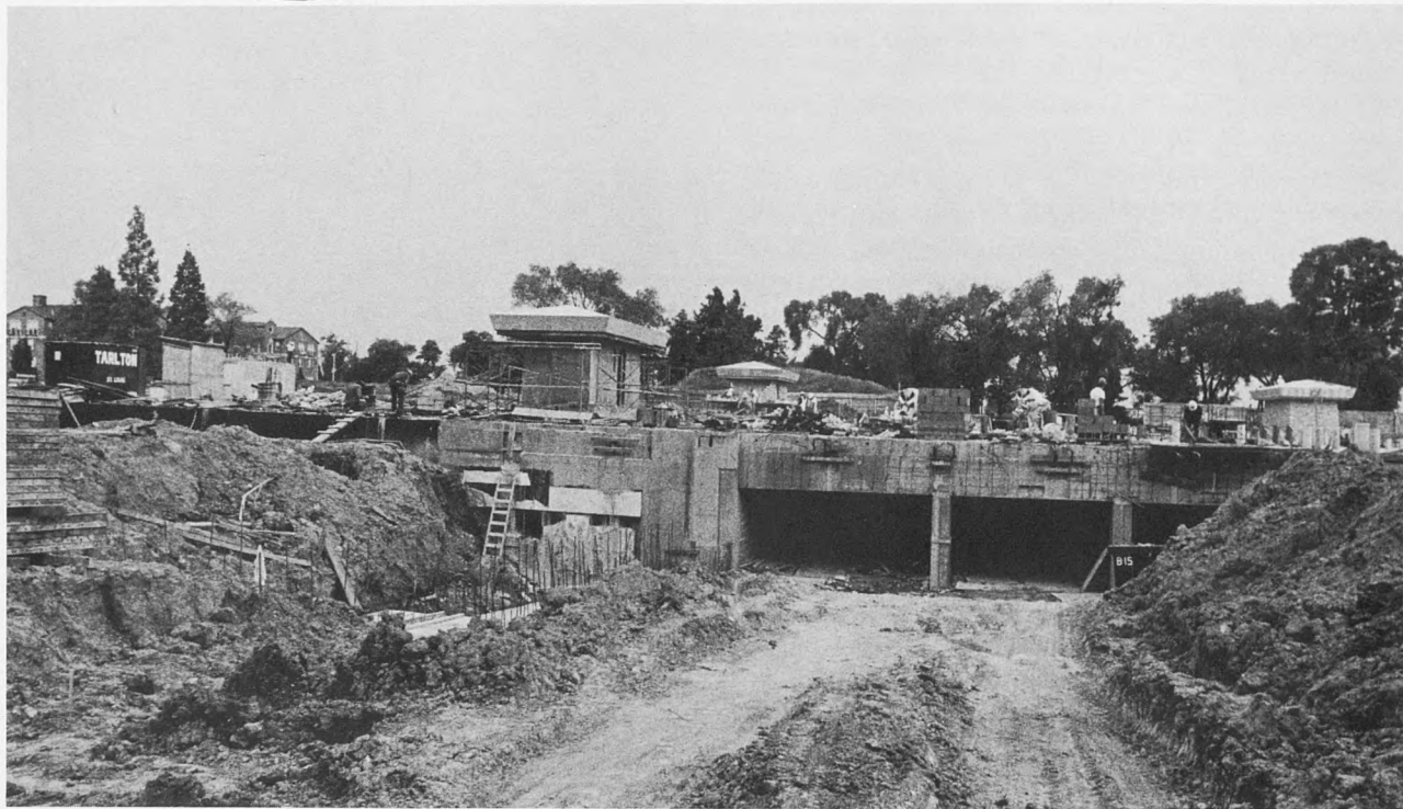
Work on the underground garage is nearing completion. The 1200-space facility is expected to be ready for
