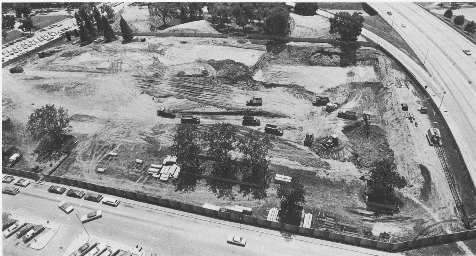
A view southward from the roof of Queeny Tower shows work progressing on the underground parking garage which is scheduled to be completed in 18 months. The street at right is Kingshighway.
