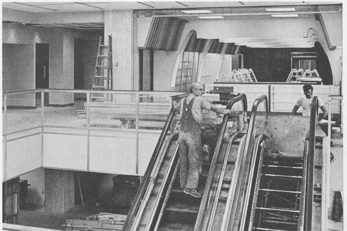
Workmen are currently completing the installation of escalators between the ground and first floor main lobby area of the new East Pavilion. The Auxiliary's Wishing Well will be located immediately behind the escalators in the area with the arch-shaped walls.
