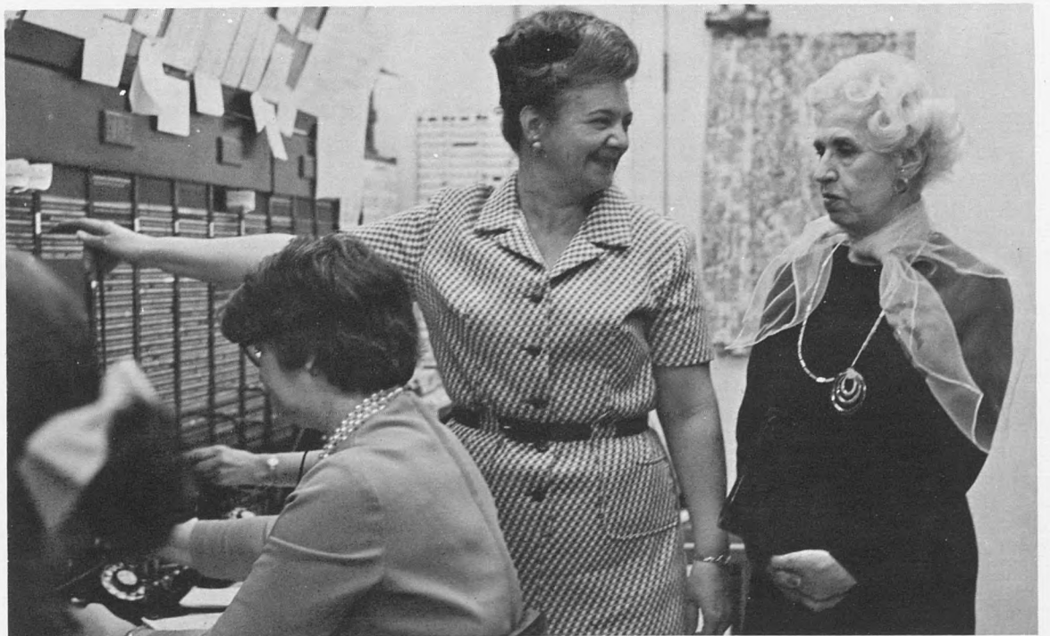
Many changes have occurred in the operation of the Barnes Hospital telephone switchboard during the past 36 years that Miss Rose Tullmann, right, has been employed in the communications department. Miss Tullmann recently requested that she be relieved of her supervisory duties as chief telephone operator and be given a transfer. Miss Tullmann will continue her work in a business and clerical capacity in the communications department. Discussing equipment changes with Miss Tullmann is her replacement, Mrs. Agnes Bardot, who was formerly a telephone operator at the hospital.
