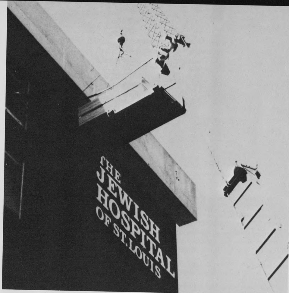
During construction of the two new Shoenberg floors in 1978, cranes and lifts were used to carry materials up to roof.
