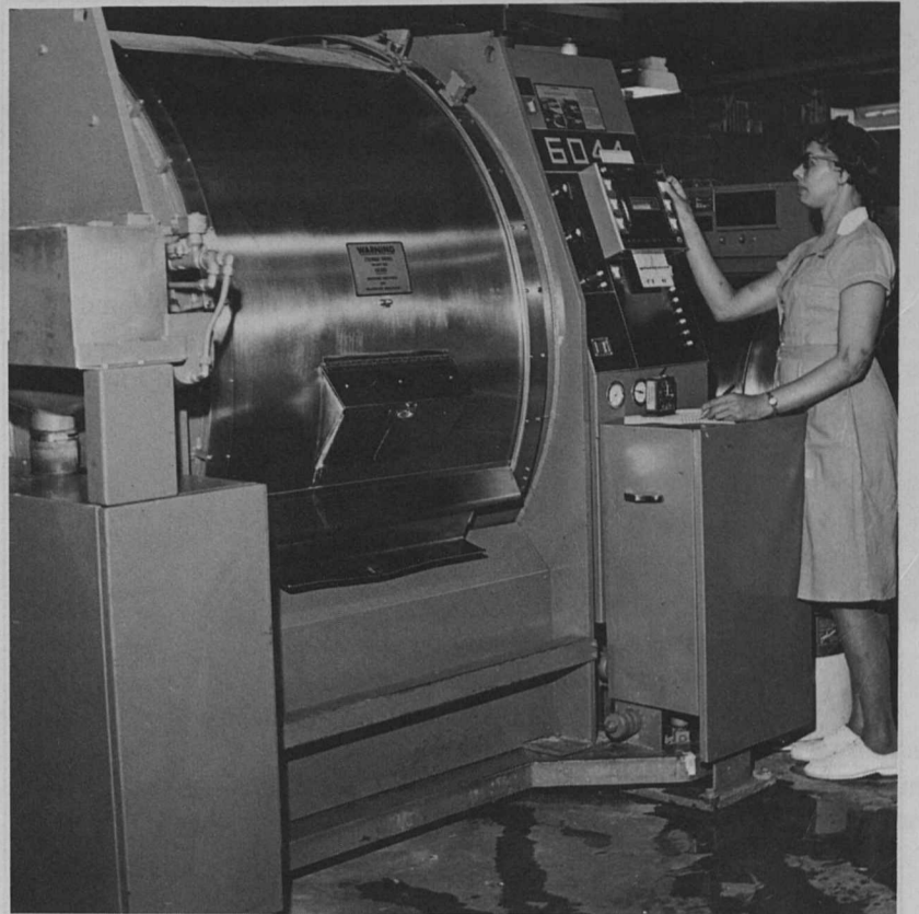
The Hospital laundry has entered the computer world with the recent addition of three new 400-pound washerextractors and modernized folding equipment. With the installation of the new machines over 8,000 pounds of laundry can be handled in a much easier and faster method. Checking out the computer on one of the new washers is Mrs. Georgia Mae Naylor, Utility Worker Grade 4.
