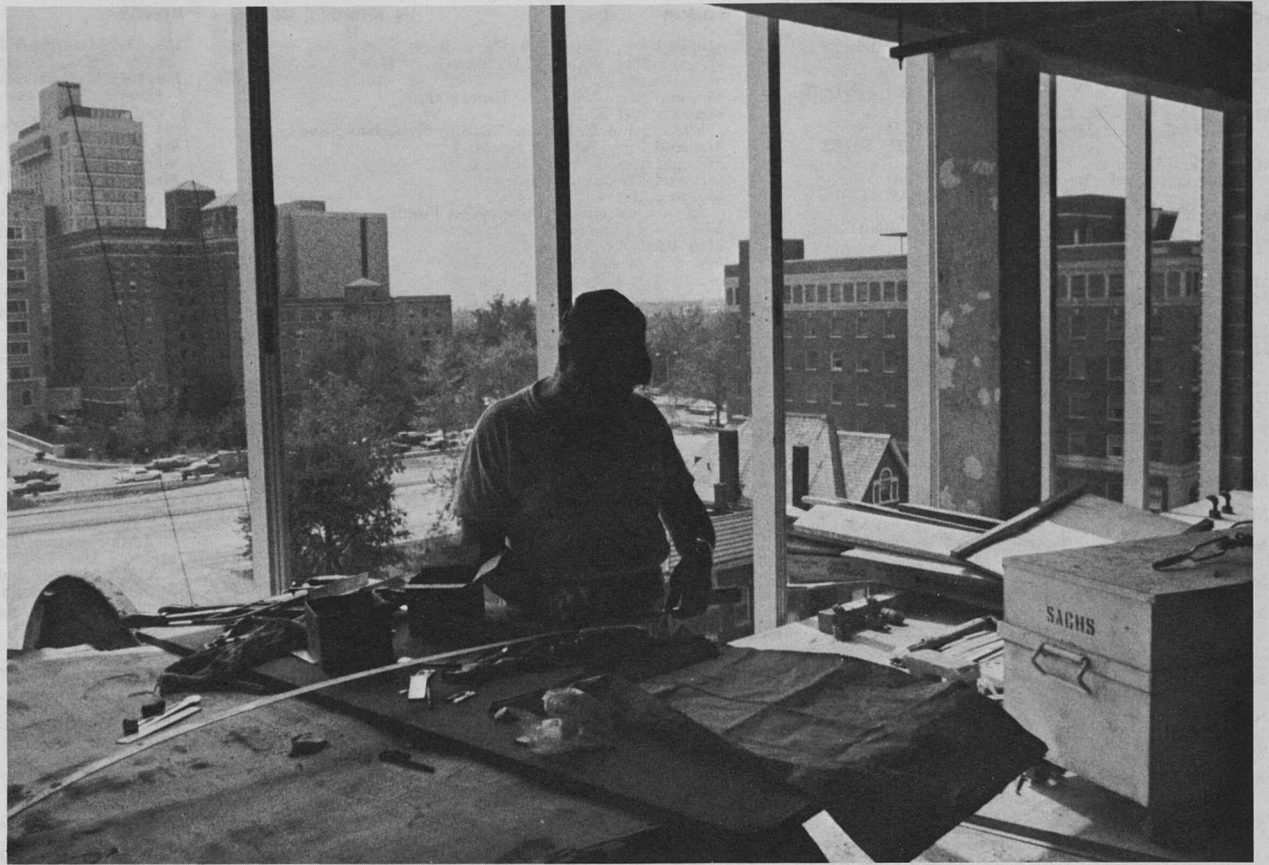
A METALWORKER ON THE SIXTH FLOOR of the Yalem Research Building is framed by the vertical metal bars which will cover the entire southern side of the building. The Moses Shoenberg Memorial Nurses Residence can be seen in the background to the right.
