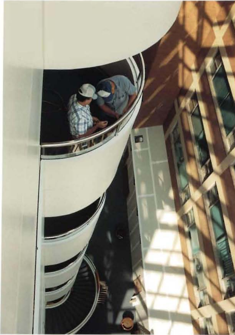
Construction workers put the finishing touches on the new Library and Biomedical Communications Center. Readers will get a closer look at the new library in a future issue.
