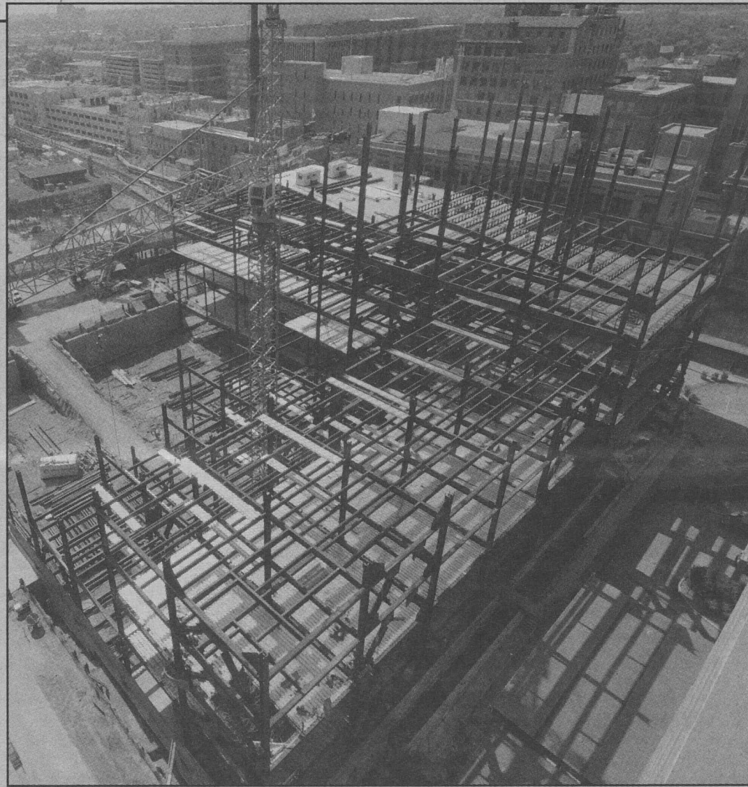
Rising to the sky The steel frame of the BJC Institute of Health at Washington University continues to rise and expand across the two-acre construction site. Crews are setting what will amount to 8,210 tons of steel by November 2008. They also are excavating a tunnel road under Euclid Avenue, which will lead to the future loading docks and will connect with Taylor Avenue. The 11-story, 700,000-square-foot building is scheduled to open in December 2009 and will be the hub for BioMed 21. Barnes-Jewish Hospital also will have five floors in the building for support services.
