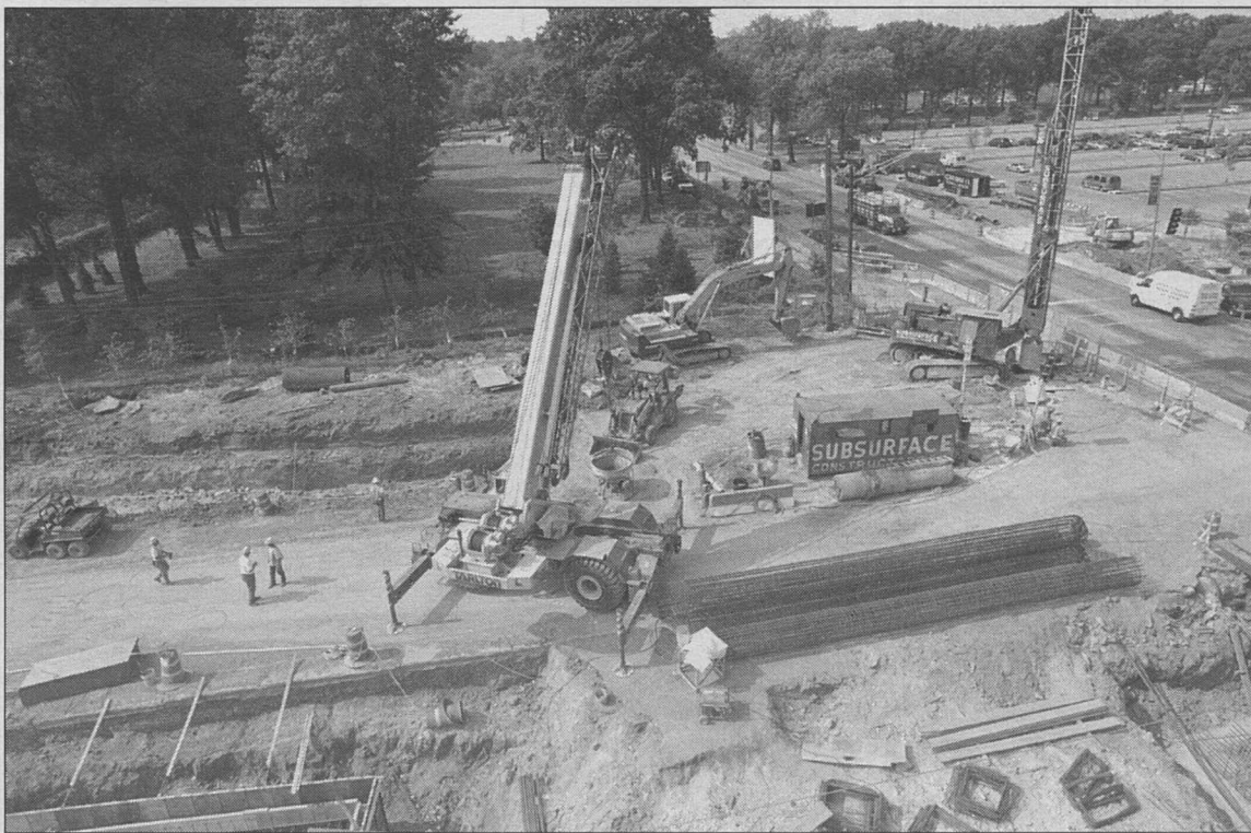
MetroLink construction at Skinker Boulevard and Forest Park Parkway — as seen above, looking south from the roof of the 276 N. Skinker Building — has continued this summer, as it has at numerous other St. Louis-area sites. Already served by a MetroLink station at the Medical Campus, the University will further benefit from three new stations: at Skinker and the parkway; at Big Bend Boulevard and the parkway; and at West Campus, at the parkway and Forsyth Boulevard.
