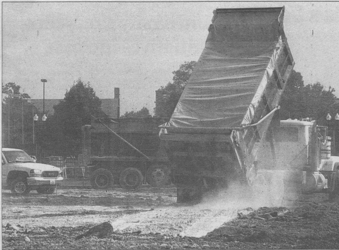
Construction crews July 19 work to perfect the soil grade that will be underneath Francis Field's new FieldTurf, a synthetic playing surface. The actual FieldTurf is expected to be installed in early August, and the project is scheduled to be complete by the middle of that month. "The field will provide a safe and consistent playing surface usable seven days a week for student-related athletic and recreational programming needs," says John M. Schael, director of athletics.
