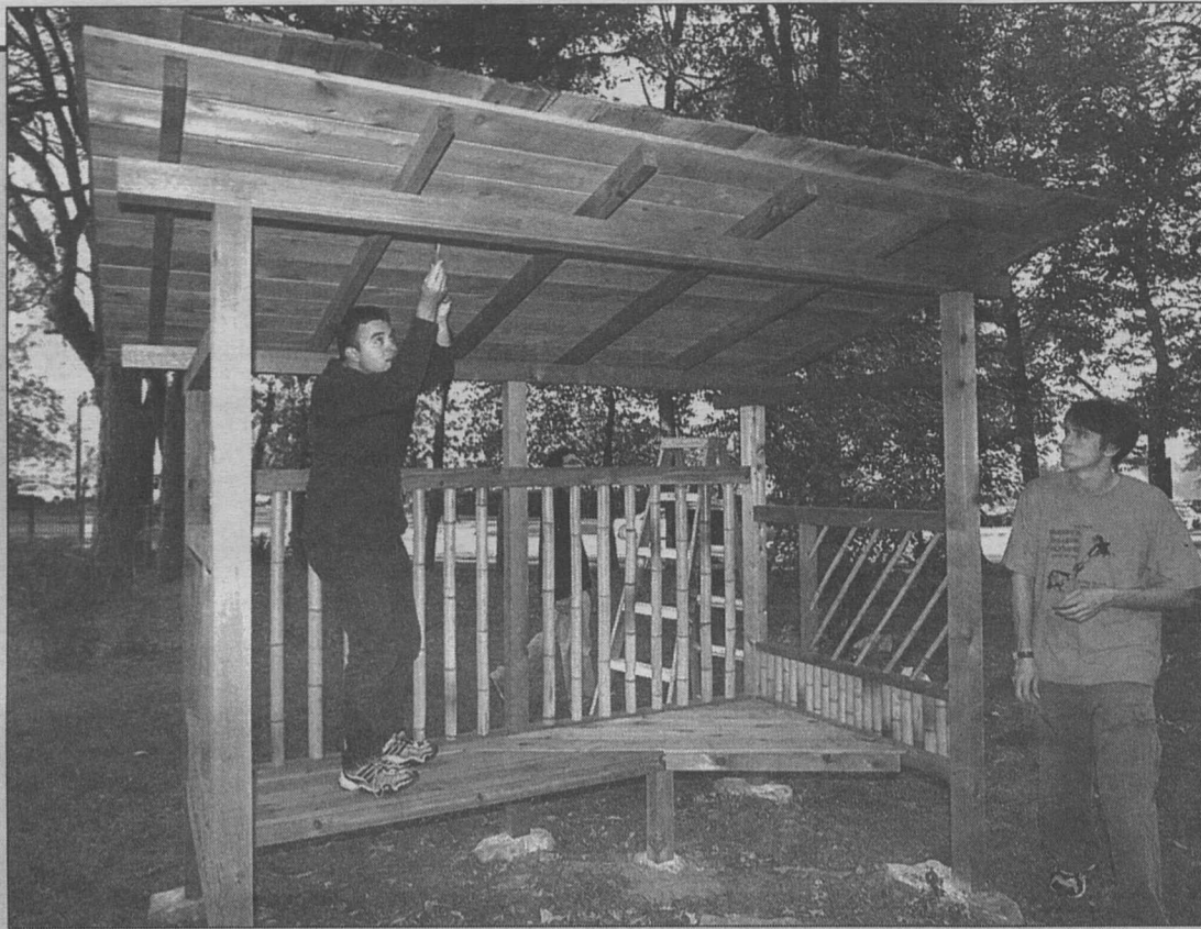
A roof over your head School of Architecture students Jordan Thompson (left) and Shawn Walsh apply finishing touches to the roof of a "koshikake machiai" — a traditional Japanese tea-house waiting bench — in the Elizabeth Danforth Butterfly Garden. They and other architecture students constructed the bench with guidance from Japanese master carpenter Tamotsu Edo, whose visit was sponsored by the Visiting East Asian Professionals Program in Arts & Sciences and the School of Architecture.
