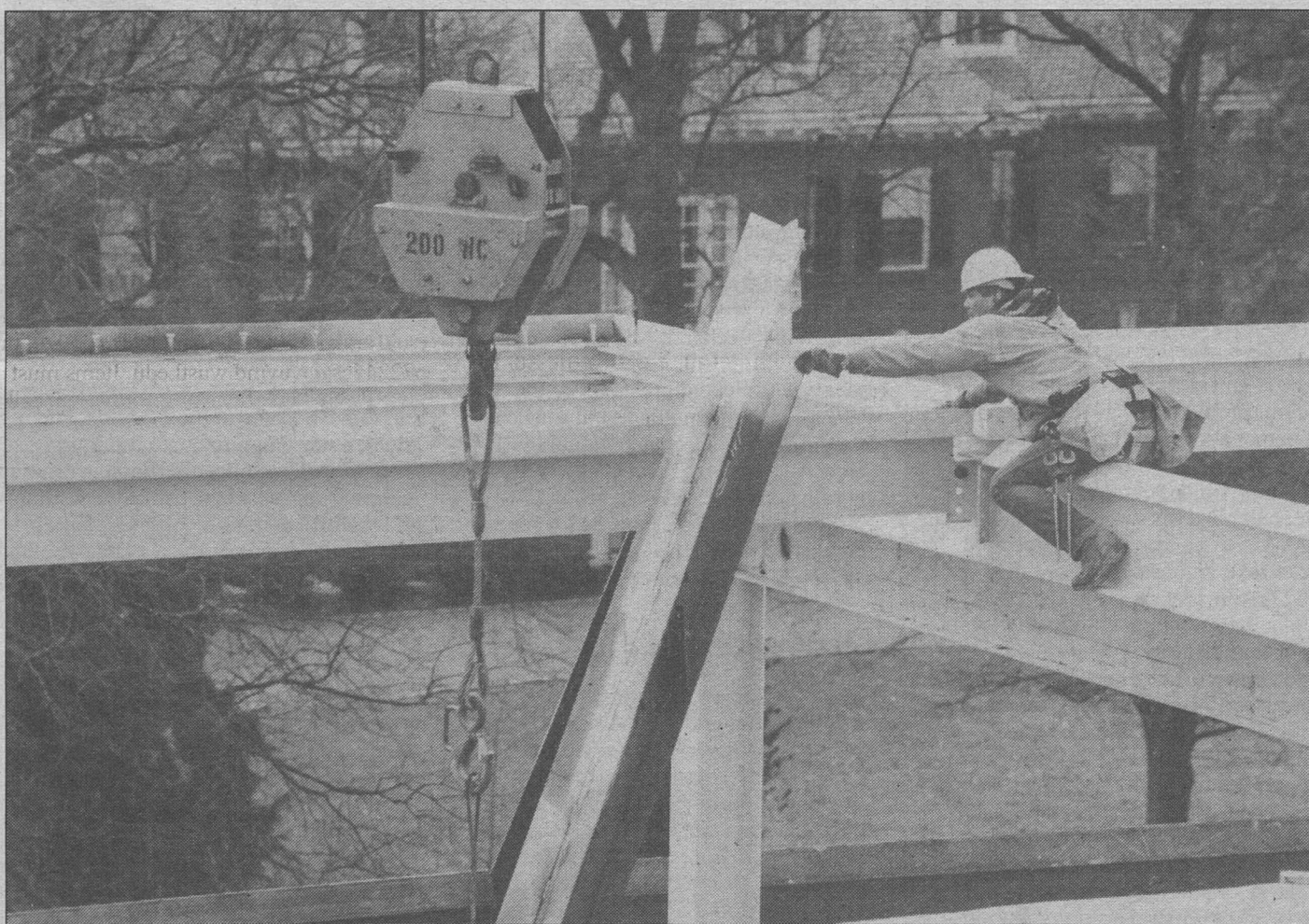
An ironworker for BSI Constructors Inc. helps set the structural steel for the roof of the new psychology building. Construction, which is on schedule, is expected to be completed in fall of 1995.
