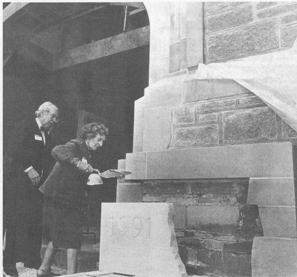
A strong foundation: Stanley and Lucy Lopata recently participated in cornerstone-laying ceremonies for the Natural Sciences Building, which is being constructed just south of Wilson Hall. Stanley Lopata is chair of the Natural Sciences Building committee and an emeritus trustee. The Lopatas have given generous contributions to many campus programs and construction projects. The new building will provide research and office space for the Departments of Biology and Earth and Planetary Sciences, as well as classroom and lecture space for other University departments and schools. Construction will be completed by late 1992.
