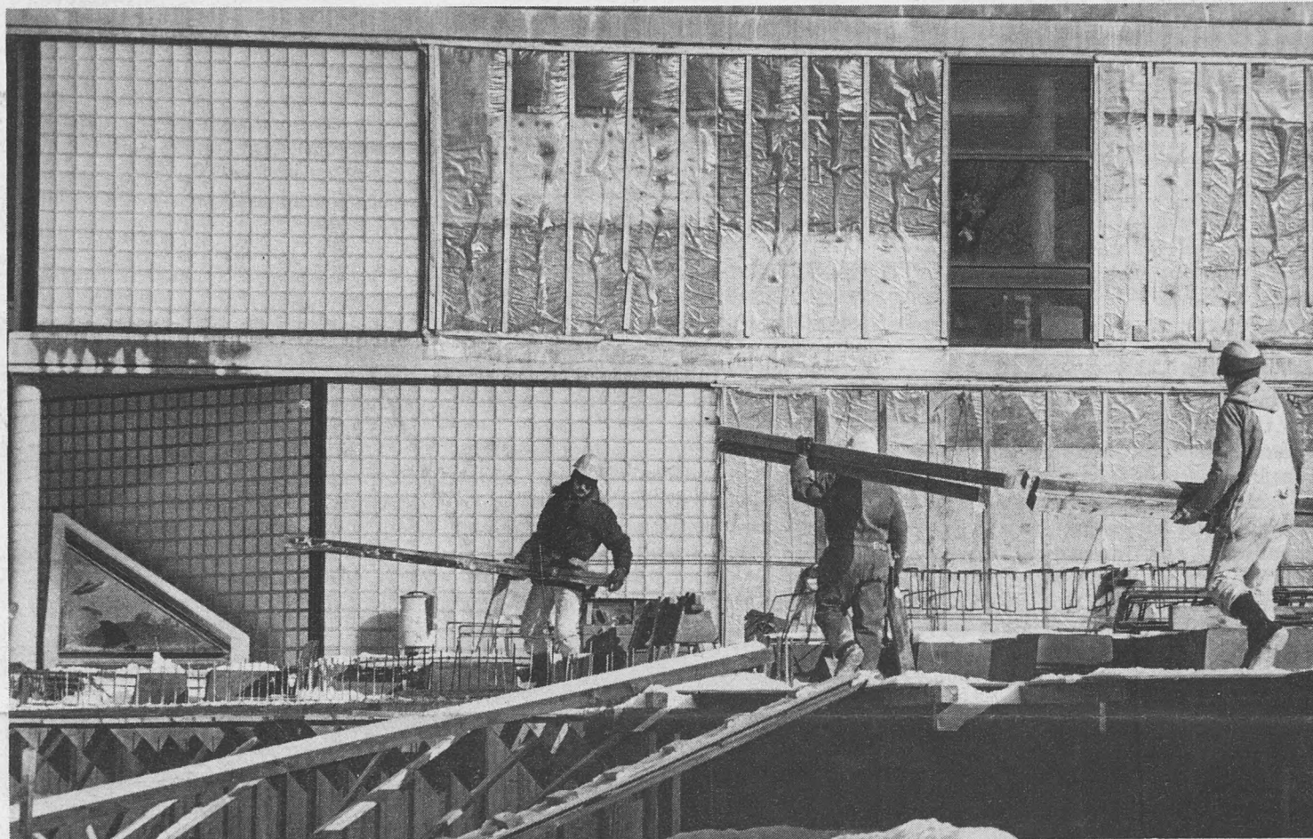
With the exception of a few days when temperatures plunged below zero, workmen were busy throughout the semester break on the addition to the bookstore. Located on the south wall of Mallinckrodt Center, the addition is expected to be finished by June 1. Remodeling of the present bookstore will be completed in August.
