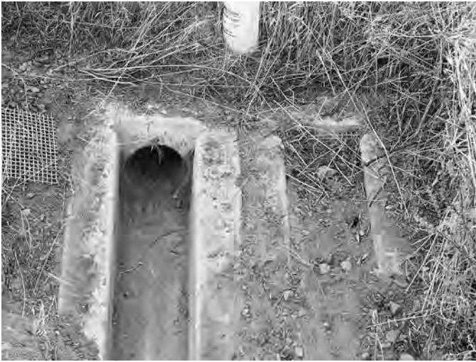
Figure 50. Dual outlets, one cleared for testing, one packed with dirt and stone, Nevada SPS-1.
