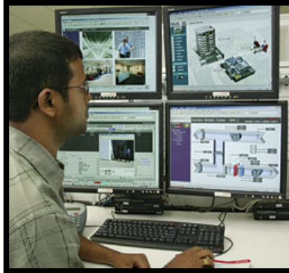
Figures 2.1.4: Example of a Honeywell Building Automation Screen View 2
