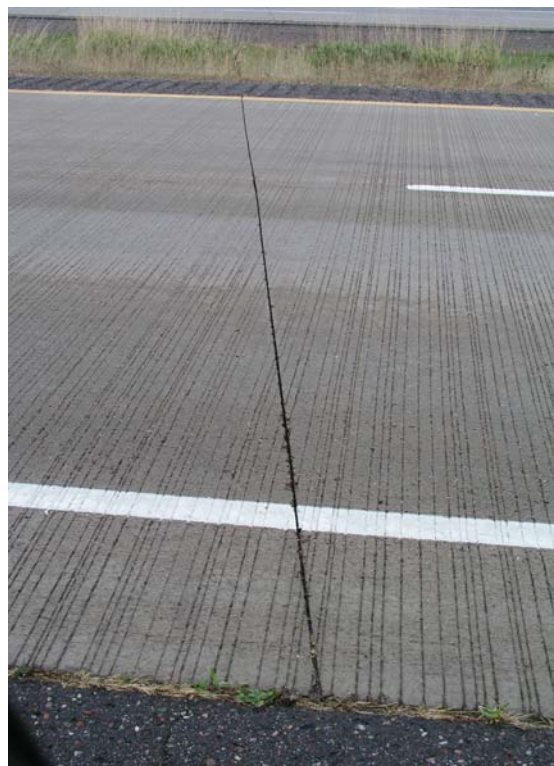
Figure 4.4.5 Typical Chipped Joint – WIS 29 Abbotsford
