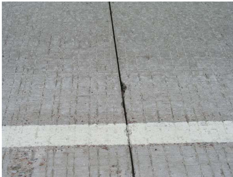
Figure 3.7: Typical Chipped Joint, November 2005
