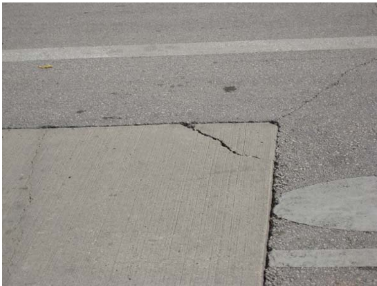
Figure 3.2: 87 th Street Bus Pad Test Section, Corner Break
