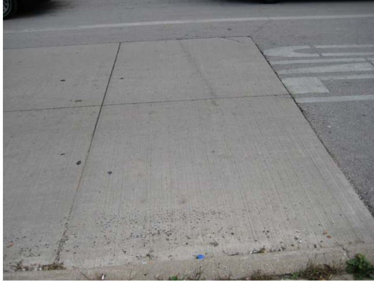
Figure 3.3: 87 th Street Bus Pad Test Section, Corner Breaks and Shrinkage Crack
