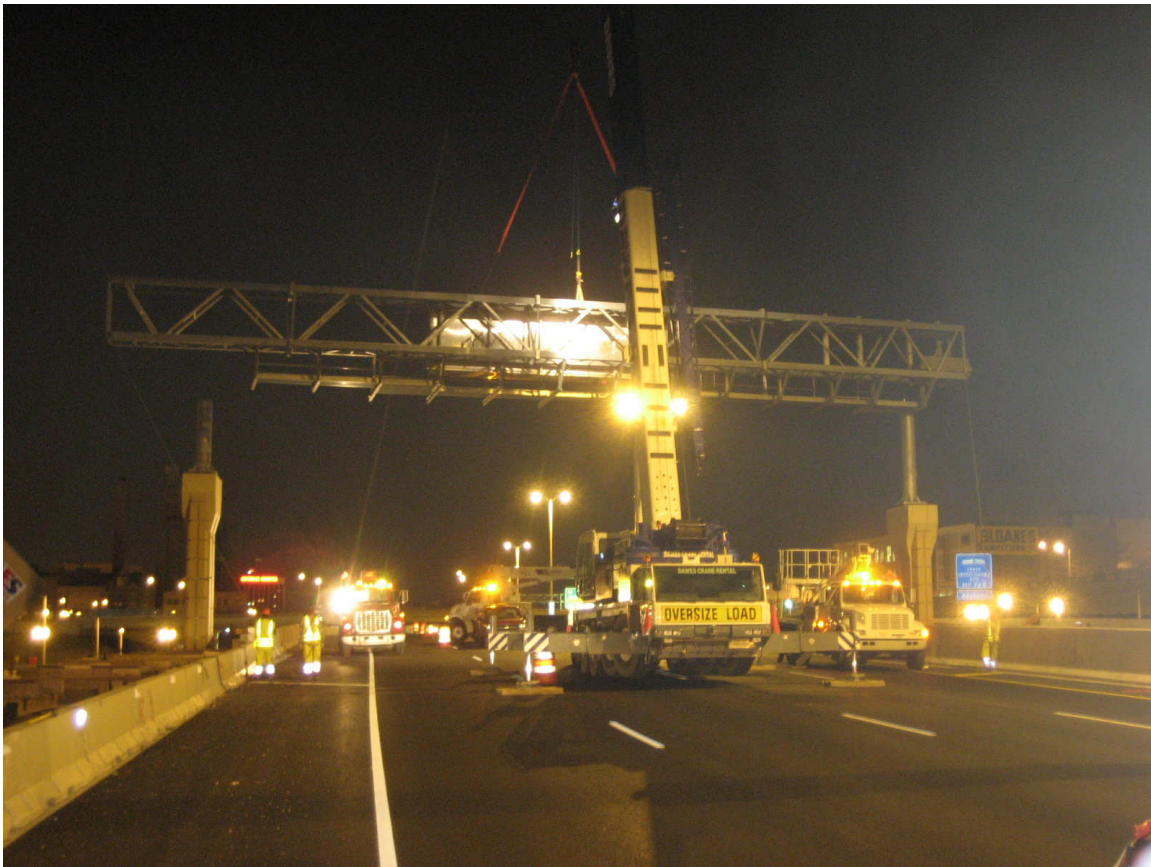
Figure 5-3 - Heavy lift crane lowering the sign bridge into its final resting position. Note that the outriggers for the crane came close to the sensor locations.
