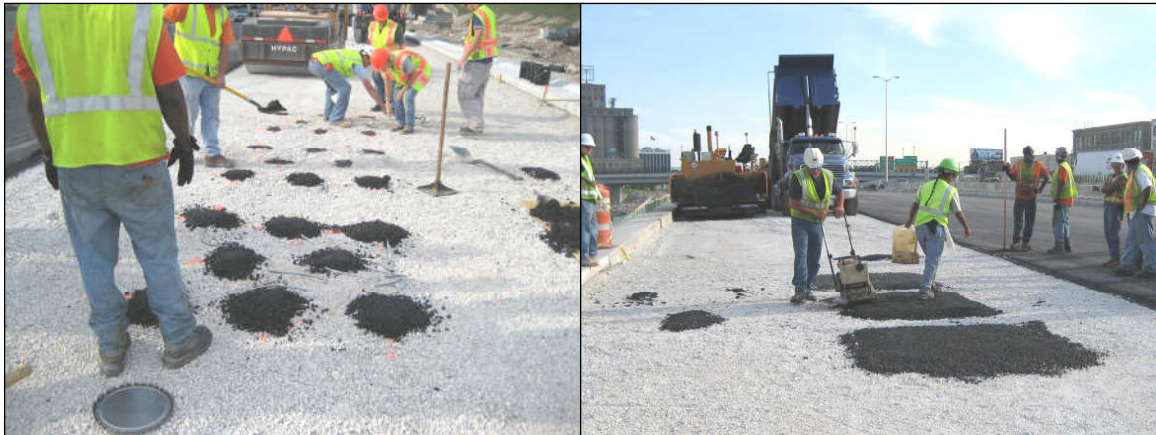
Figure 2-8 - Left: Placing screened asphalt on top of gauges and carefully compacting. Right: Compacting the unscreened asphalt over the gauge arrays with the paving crew approaching.
