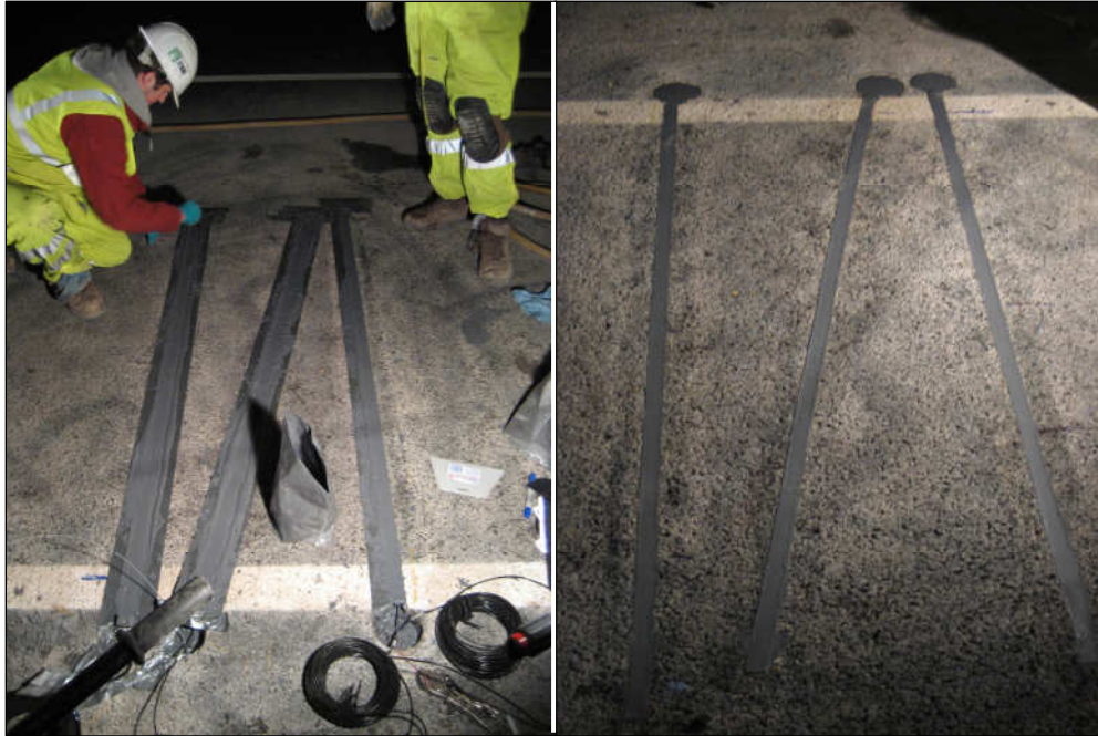
Figure 2-16 - Left: All three wheel-wander sensors have been installed and the grout on the final sensor is being leveled with the pavement surface before hardening. Right: All three sensors installed with the tape removed.
