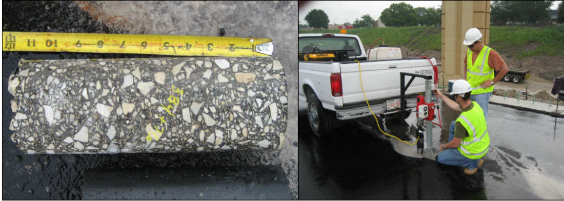
Figure 5-2 – Left: Core sample removed from the pavement. Right: The core-drill was secured against the weight of a vehicle to produce samples with very smooth side walls for possible future testing.
