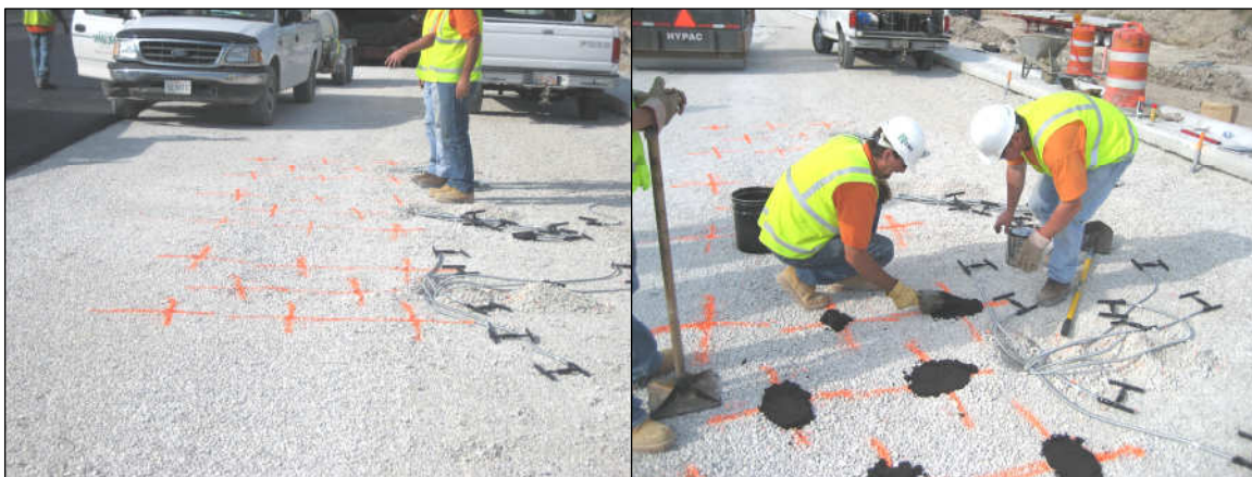
Figure 2-7 - Left: Marking the proposed locations of the gauges. Right: Placing sand/binder pad and fitting gauges.
