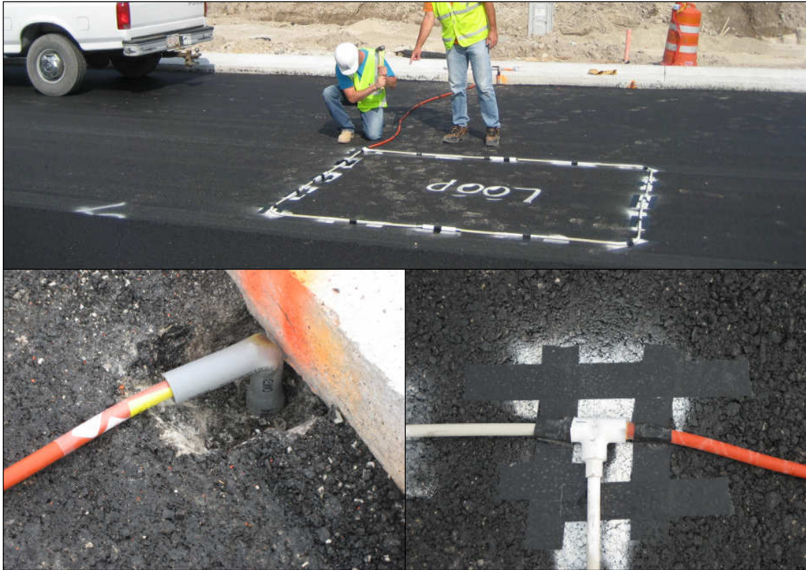
Figure 2-10 - Pictures showing various parts of the loop detector installation. Top: The fiberglass tape was hammered lightly to create a good bond to pavement. Bottom left: The asphalt around the conduit was removed with a cold chisel and hammer to expose enough conduit to install a “homemade” 90° elbow. The rather thick looking orange cable actually ends just inside this elbow and only two small wires actually pass through the elbow. Bottom right: A close up showing how the corner was adhered to the pavement and also the construction of the Never Fail Loop.
