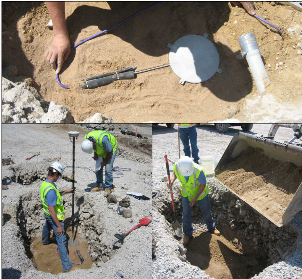
Figure 2-3 –Top: Placing EPC in a bed of fine sand and routing sensor cable carefully. Bottom left: Measuring and recording the final location of the EPC with a GPS based measuring device. Bottom right: Backfilling against the EPC with sand.
