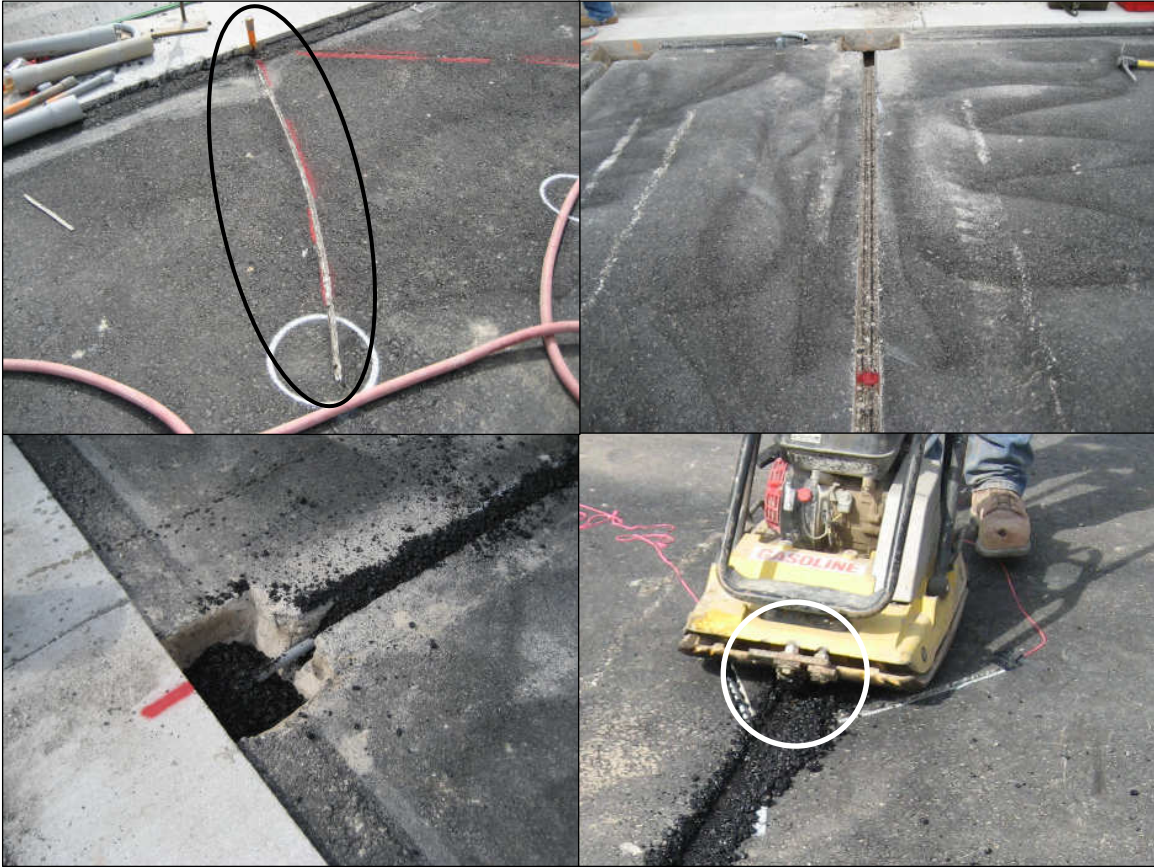
Figure 4-3 - Installation of the WIM, wheel wander, and temperature sensor conduits. Top left: Grooves were cut with a saw for the sensor leads for the pavement temperature gradient probes. Top right and bottom left: Groove cut with conduit in place for a WIM sensor. Bottom right: Asphalt being re-compacted into groove cut for the wheel-wander sensors. The plate tamper had a bolt-on bar (circled) mounted on the bottom to fit into the cut to increase compaction efficiency.
