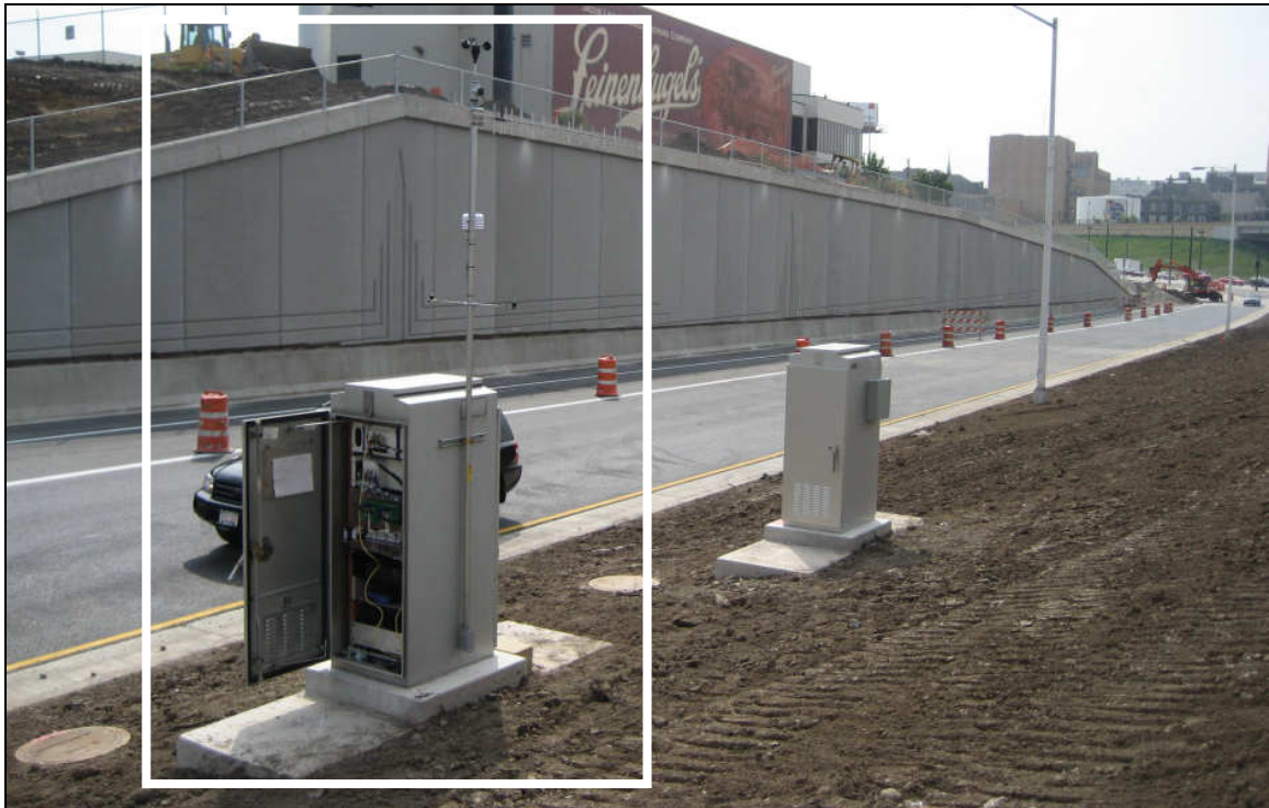
Figure 2-11 - The highlighted cabinet is occupied by the equipment for this project. The mast connected to the cabinet holds environmental sensors as well as the wireless communications antenna. The cabinet in the background houses various traffic control devices for WisDOT. The two cabinets are connected by a limited number of conduits.
