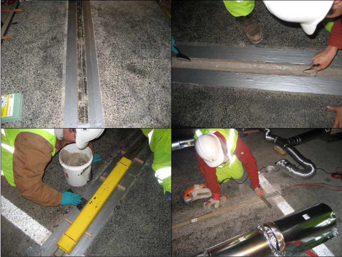
Figure 2-18 - Upper left: Channel for the WIM sensor ready for installation. Upper right: Grout for the sensor being distributed into the channel. Lower left: Sensor in place with pieces of steel placed across the leveling beams to keep sensor from floating out of the grout. Touch up work to the grout was done before its initial set. Lower right: The sensors were ground flush with the surrounding pavement and checked using an 18-inch long straight edge.
