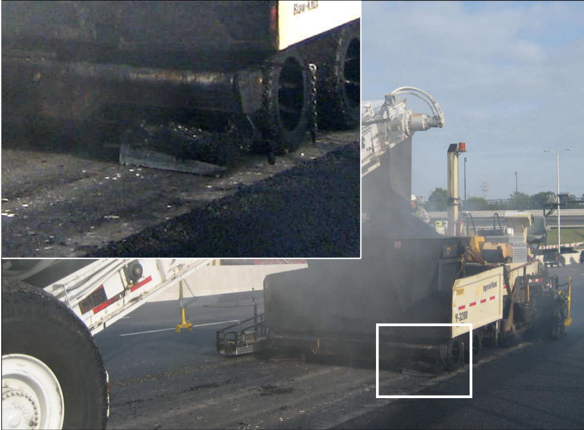
Figure 2-14 – The scraper in the wheel paths of the pavers should be lifted off the pavement surface to avoid destroying sensors and their wiring. The inset picture is a close-up of the scraper which is in the down position, resting on the pavement surface.
