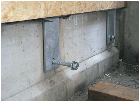
Fig. 15 Connection of the wall element with the foundation by means of steel angles
