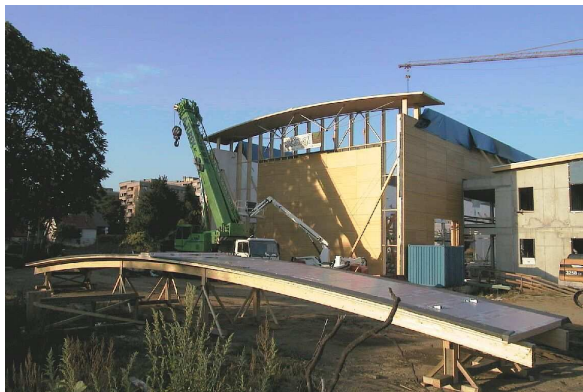
Fig. 12 First roof element at the final position and assembling of the second element at the ground
