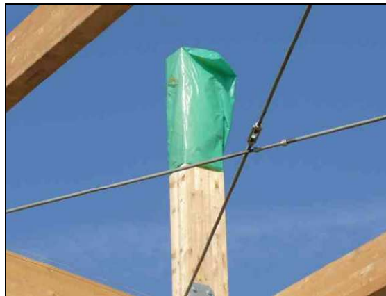
Fig. 11 Weather dumping protection of a column element
