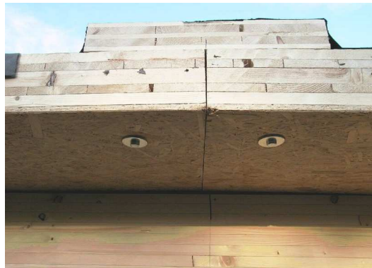
Fig. 23 Joint of the roof's CLT-plates by means of an overlap with a 5-layered CLT-strip
