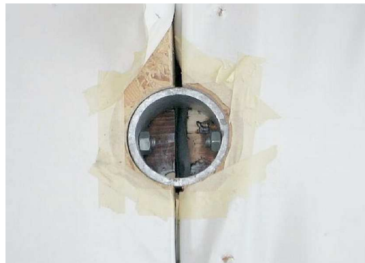
Fig. 16 Connection of the wall elements with special cylindrical steel fasteners with glued-in rods
