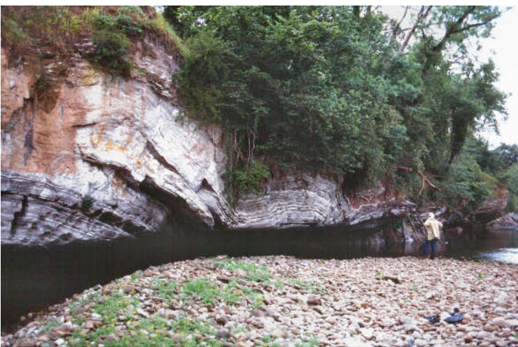
Figure 6. The gypsum cliff in 1990 just before it collapsed showing the complete flow of the River Ure going under the face.
