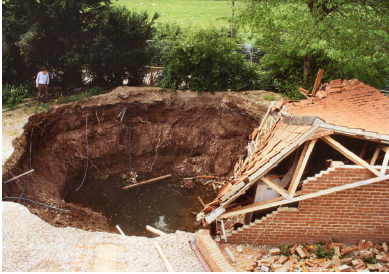
Figure 12. The Ure Bank Terrace collapse in late April 1997 viewed from the upstairs window of the house.
