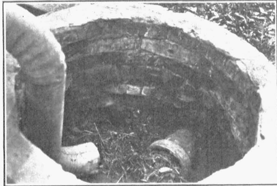
FIG. 8.—Filter without filtering material and with trash in pipe.
