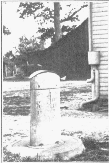
FIG. 6.—Cistern with metal top. Filter shown on wall helps but is too small.
